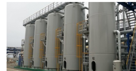
Activated carbon filtration facilities
